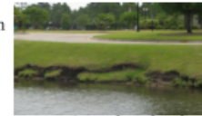
An eroding shoreline.
