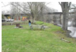
Minor shoreline erosion that can be resolved with plantings.
