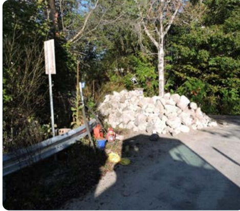
Clean, washed rock is stockpiled before being loaded onto a crane bucket to lower into the spawning bed.
