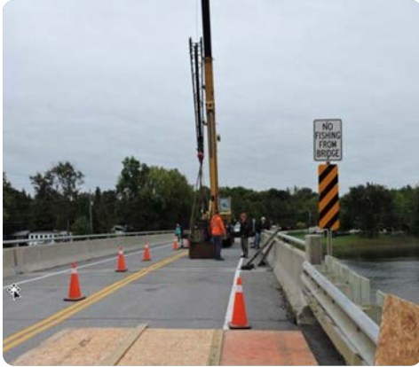
Crane being set up to lower rock to walleye spawning bed from a bridge. (Plywood protects the road.)
