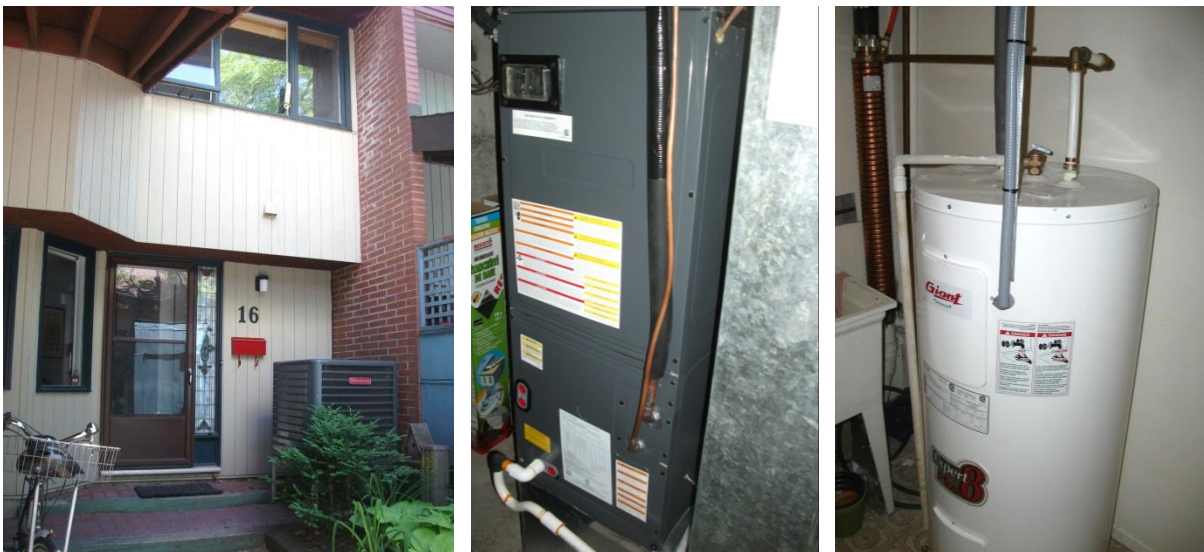
Heat pump, air handler and water heater with drainwater heat recovery unit
