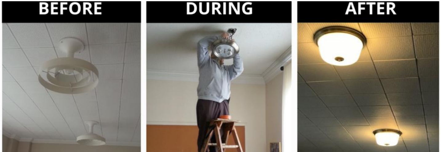
Before and After results of Palmerston United Church replacing light fixtures and installing LED lights.
