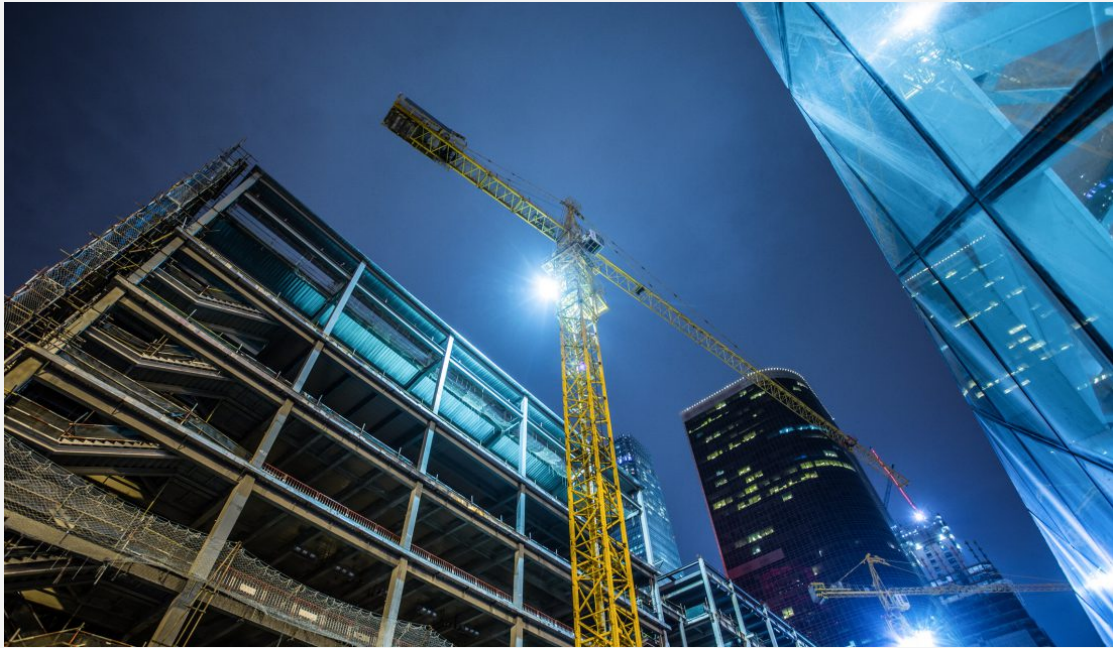
The light from ongoing construction can disrupt species' feeding or breeding behaviours.
