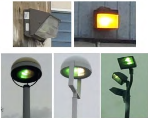
Figure 1: Existing lighting systems [3]
