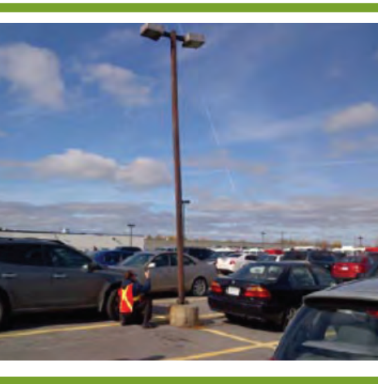
Figure 1: Post top lighting fixtures before project - Employee parking lot (2)
