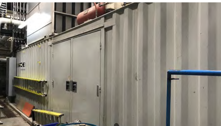
Figure 1: 1 MW Cogeneration System [3]
