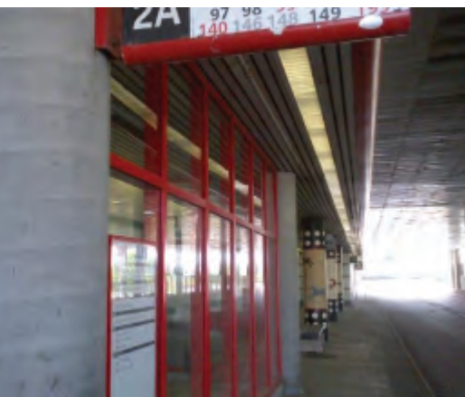
Figure 1: Existing fluorescent strip luminaires (2)
