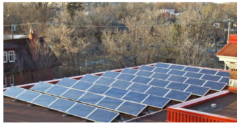
Figure 1: Rooftop Solar Installation at Muchmore Public School [5]
