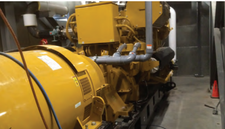
Figure 2: The Cogen Engine [5]
