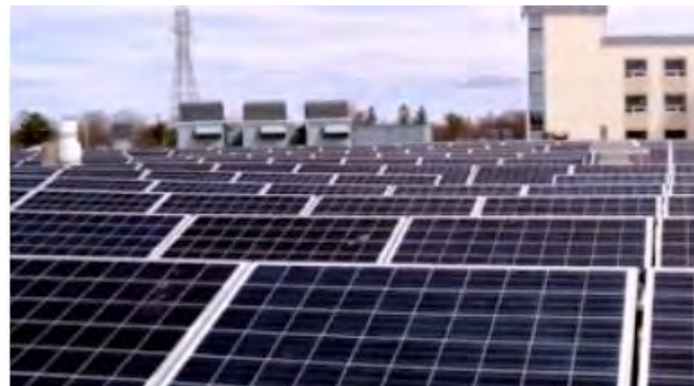
Figure 2: Rooftop solar installations at the Perley and Rideau [4]
