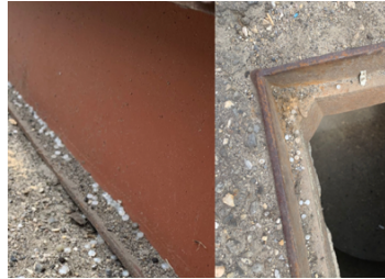
Figure 3 shows the litter in and around the catchpit prior to the LittaTrap installation
